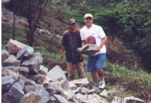
Jerry Fonner, right, donning his KVS T-shirt, assists a local mason with building the foundation of a new home.
