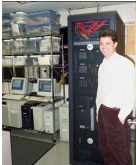
Jerry Fonner displays the new server rack beside him in the new "Tech Center" room at KVS.
